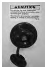
Tank Flush Inlet
